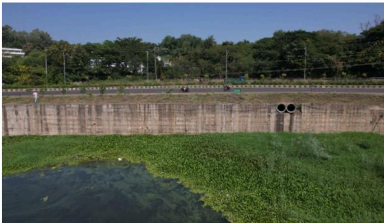
Figure 19: A sewage outlet spotted near the Kaliasot Dam
