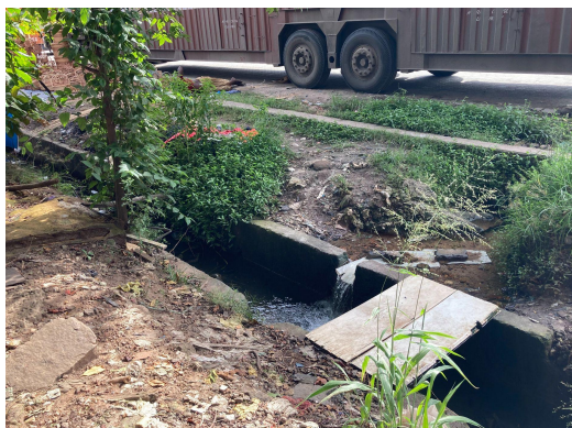
Broken municipal water pipe
