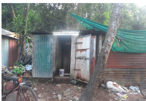
Poorly maintained common toilets
