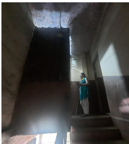
A room that has no ventilation, built on a staircase landing space
