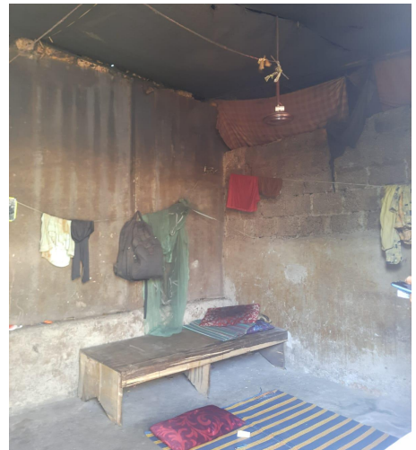
Room rented to single men, covered in soot; and a ceiling fan supported by a rope.
